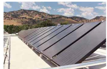
Solar water heating panels at North Boulder Recreation Center
