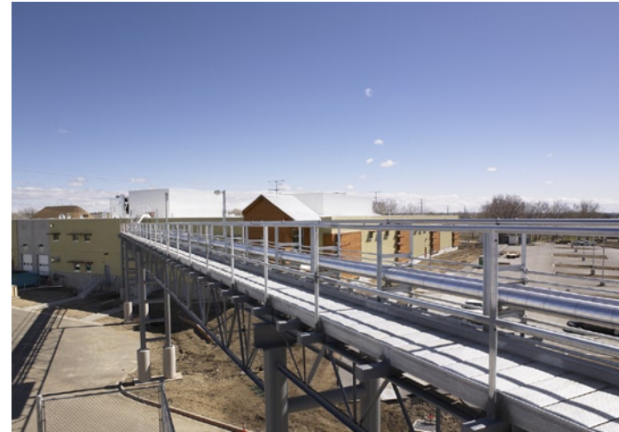
Elevated pipe bridge transports the beer.
