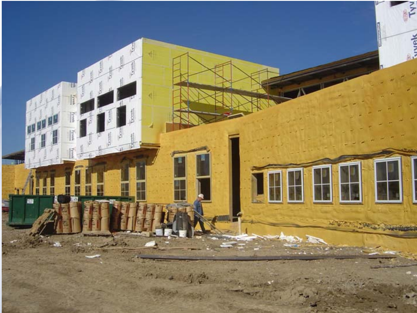
3" Sprayed-On Polyurethane Insulation
